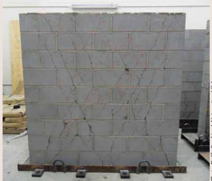
Typical wall crack pattern (outer and middle cores reinforced 15M bars, joint reinforcement every 2nd course)
